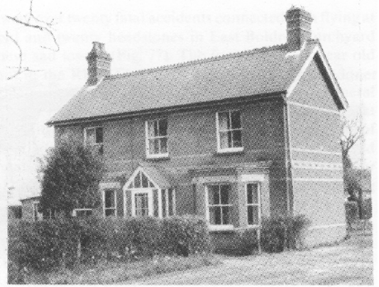
Fig. 71. Norfolk House, with missing chimney pots.
